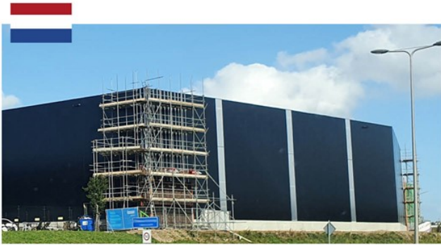
Satellogic High Throughput Plant, Netherlands
